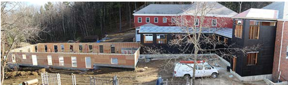
This perspective shows how the new dormitory (L) and connector are situated in relation to existing Retreat Center accommodations.
